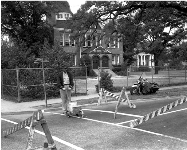
A city worker repaints crossing lines in front of the Washington School on Washington St, 1940s
