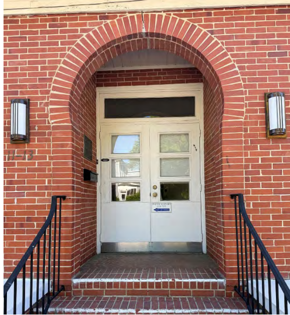
Figure 2: Proposed door to be replaced
