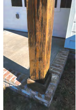
Above: Existing Front Porch Post.
