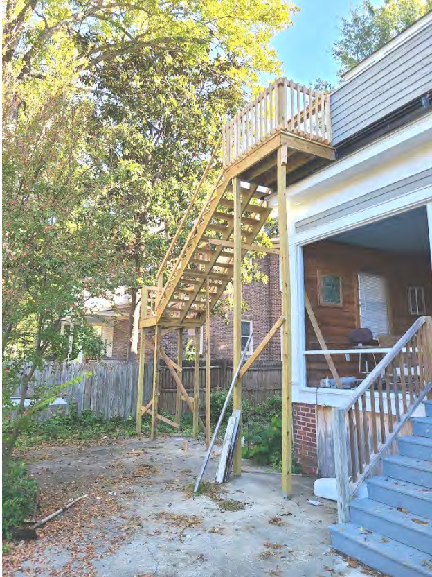
Above: Partially constructed staircase (built without permits), proposed to be removed to the upper landing and reconstructed in configuration as proposed by this application
