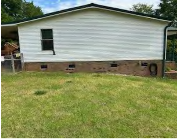
Above: Left side of dwelling as viewed from the north side of the structure
