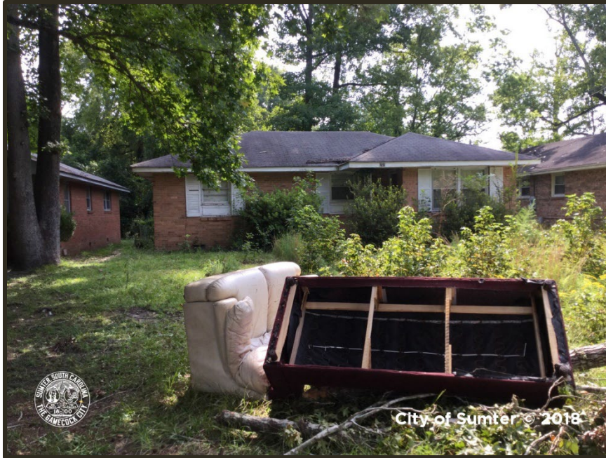
Photograph 28 Loring Example of “Poor” Condition Property
