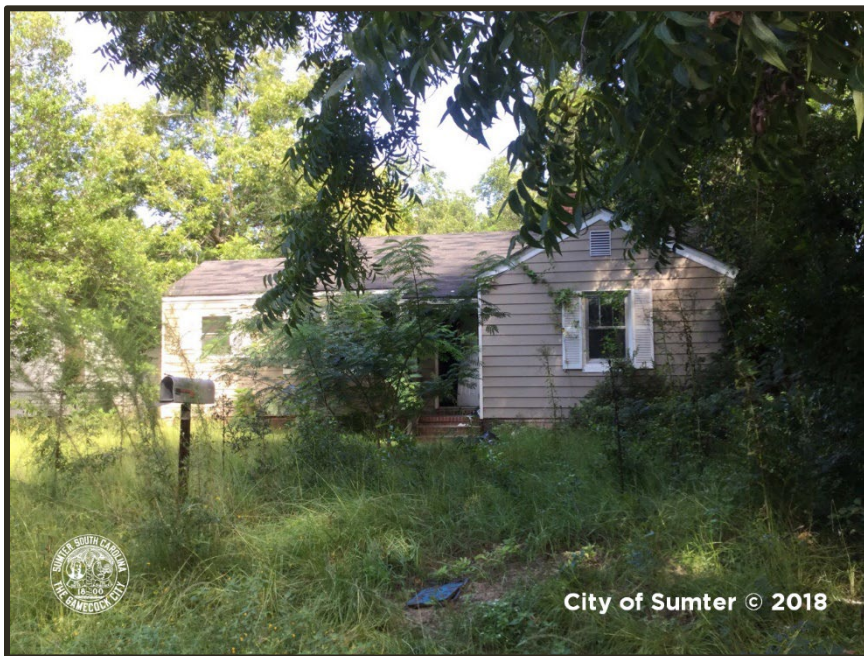
Photograph 18 Folsom Park Example of "Hazard" Condition Property
