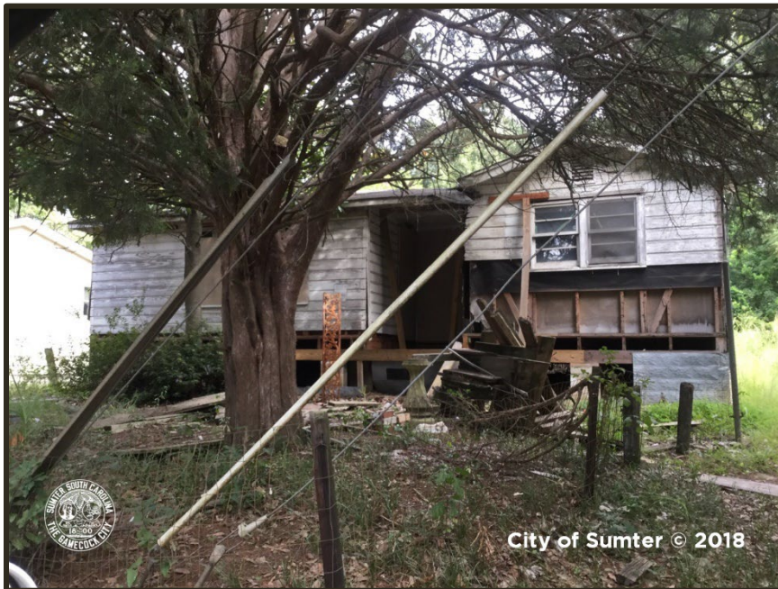
Photograph 66 Wilder Example of "Hazard" Condition Property
