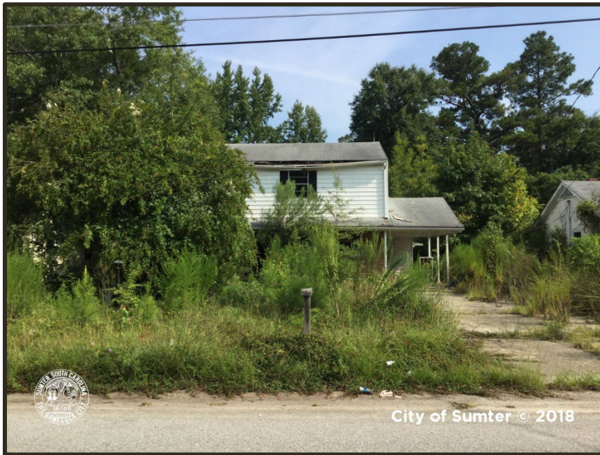
Photograph 29 Loring Example of “Hazard” Condition Property
