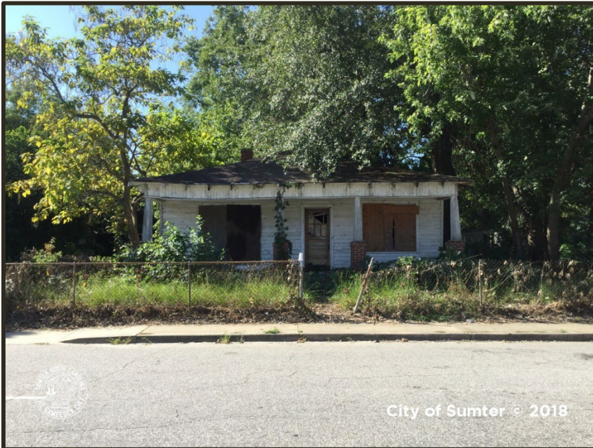
Photograph 4 Bates Example of “Hazard” Condition Property
