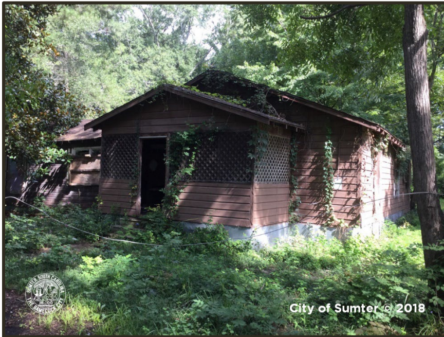
Photograph 41 Morris College Example of "Hazard" Condition Property
