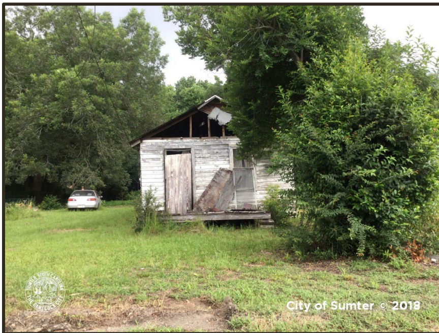
Photograph 459 Palmetto Park Example of "Hazard" Condition Property
