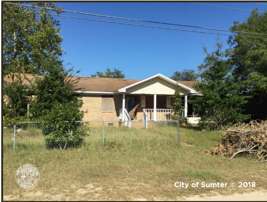
Photograph 65 Wilder Example of "Poor" Condition Property
