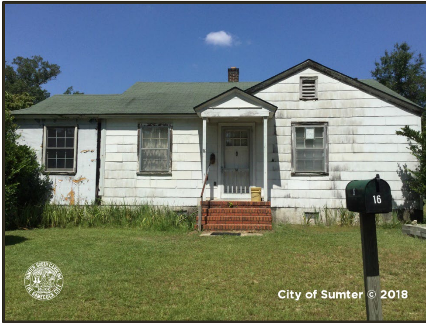
Photograph 51 Second Mill Example of "Poor" Condition Property
