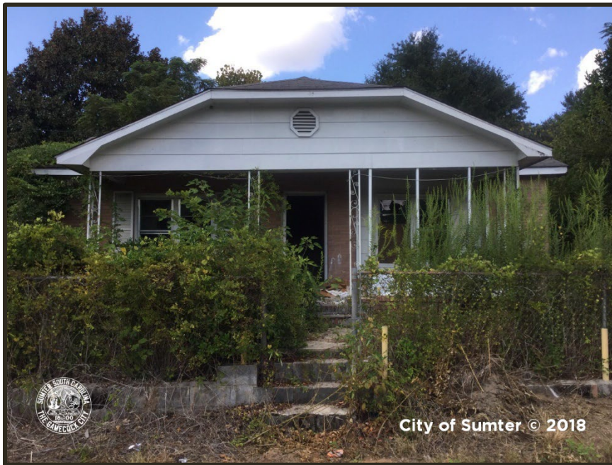
Photograph 8 Birnie Example of "Hazard" Condition Property
