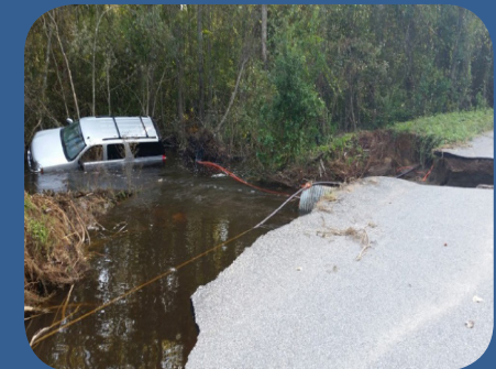
Photo: Flood Damaged Road in Sumter County
